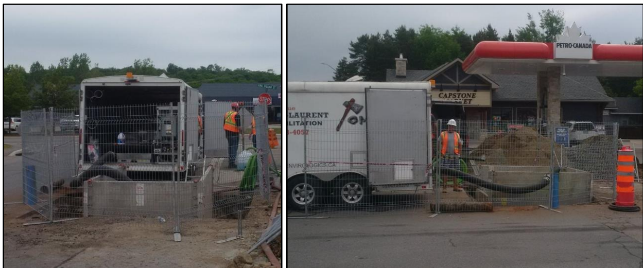
Pictures: Above, Tomahawk cleaning and lining unit set-up on Scott Street in Huntsville, Ontario.
