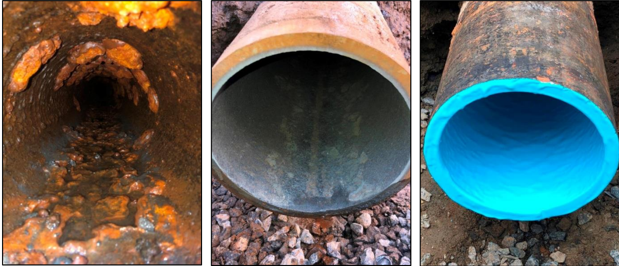
Pictures: Above left, watermain before cleaning, center, after cleaning with Tomahawk, right, after lining with Tomahawk BluKote™.
