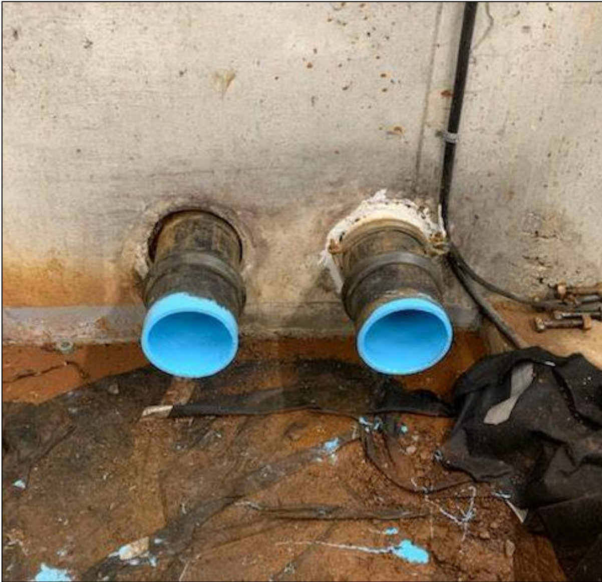
Above, both pipes after lining with BulKote™ from within the mechanical room.
