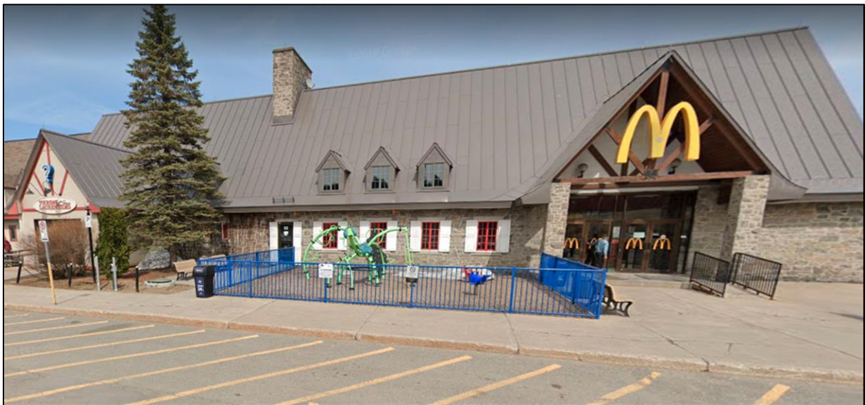
Above, worksite location of CEL water pipe rehab activities just north of Saint Jerome, Quebec.
