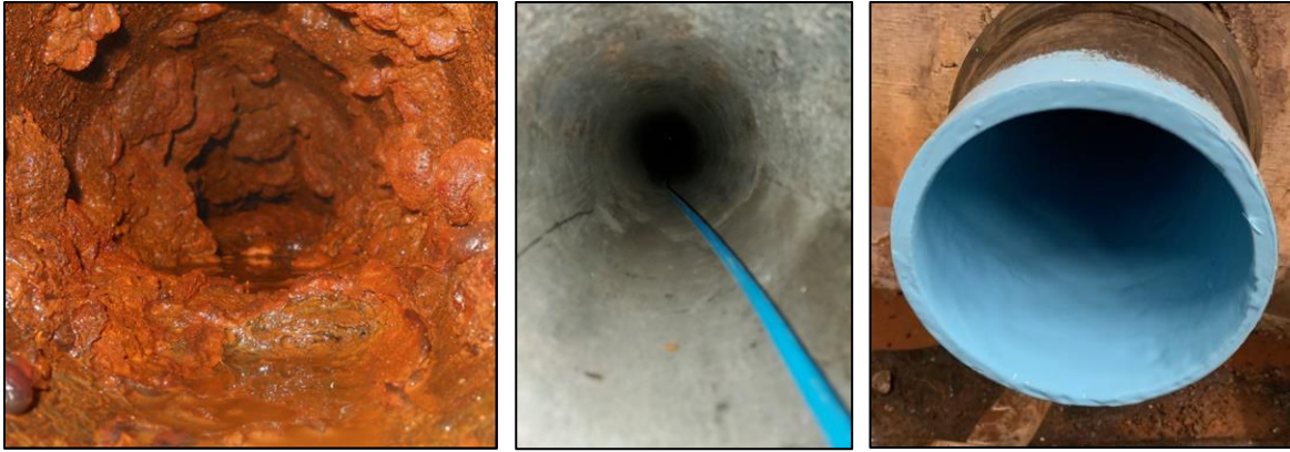
Pictures: Above left, drinking water pipe before cleaning, center, after cleaning with Tomahawk, right, after lining with BluKote™.
