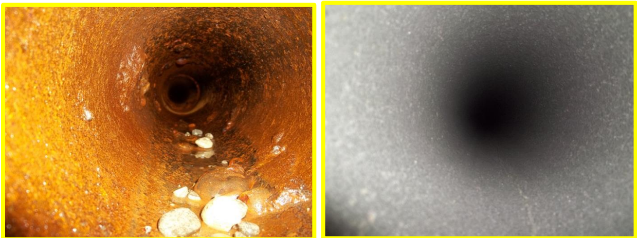
Figure 3. City of Cambridge pilot project pre and post Tomahawk™ pipe cleaning and surface preparation.
