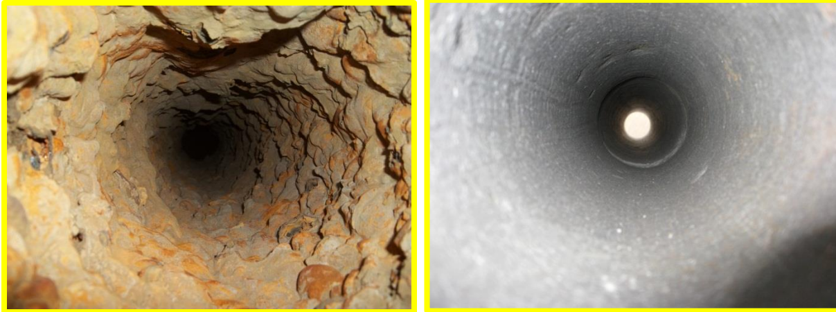
Figure 2. Pre and post pipe cleaning and surface preparation using the patent-pending Tomahawk™ System.
